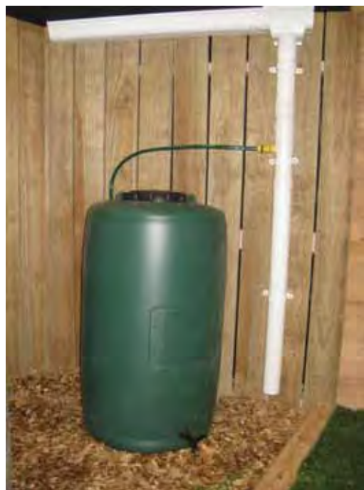
Figure 8: 250 litre rain barrel connected to down pipe via water collectors/diverter
