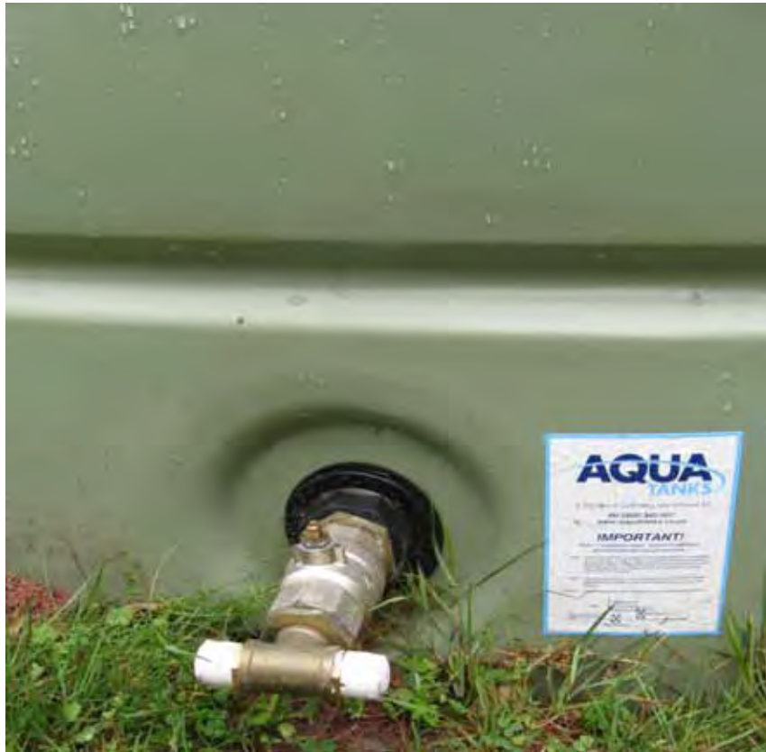
Figure 2: Emergency rainwater tank without taps at Pukerua Bay School
