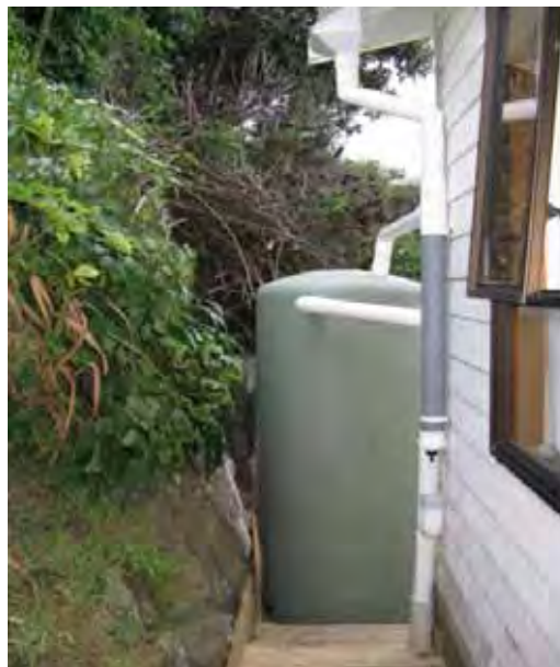
Figure 5: A 1,000 litre rainwater tank with screened rainhead and first flush diverter installed at dwelling in Paekakariki
