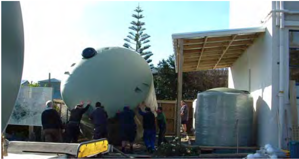
Figure 7: Unloading a 25,000 litre rainwater tank at the Roof Water Research Centre at Massey University in 2005
