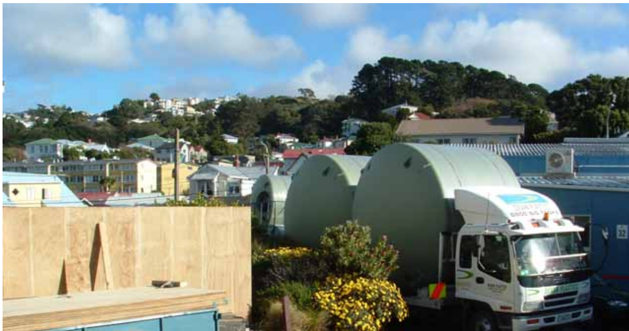
Figure 6: Two 25,000 litre and four 5,000 litre rainwater tanks being delivered to the Roof Water Research Centre at Massey University in 2005.
